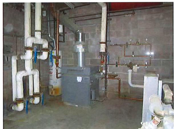
Mechanical Room South Building
