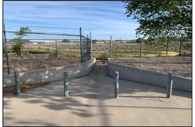
Picture 20 – Bollards and concrete scupper on the northwest portion of the Property.
