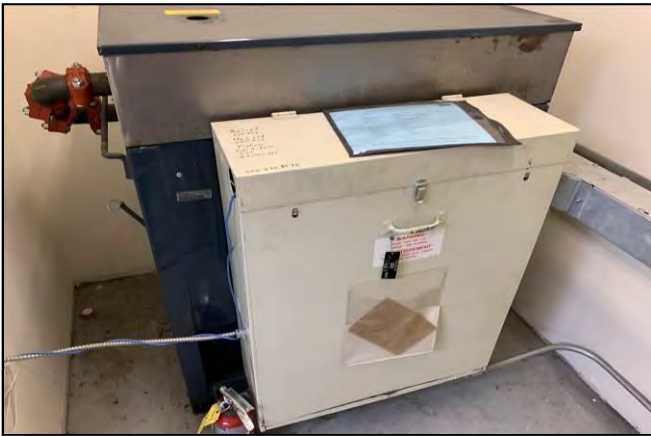
Picture 9 – Hydraulic elevator equipment within the building.
