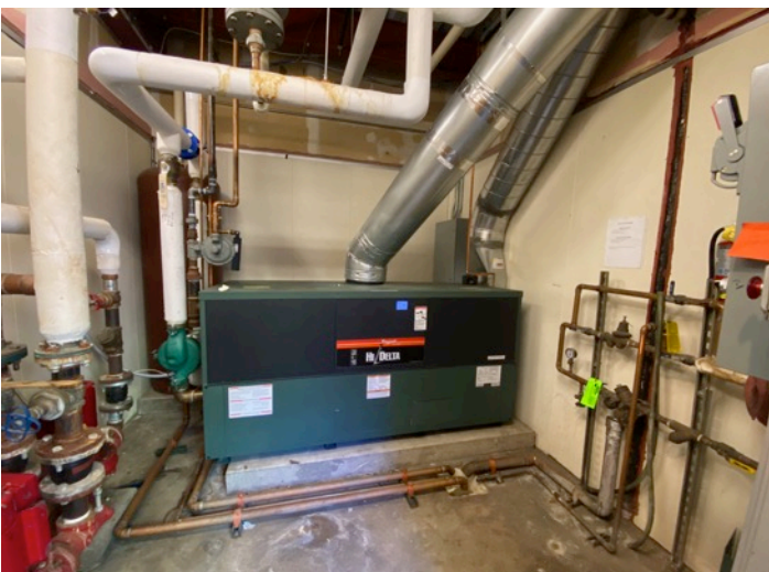
Newer boiler in first floor equipment room.
