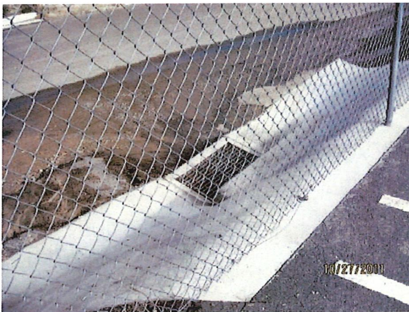
View of the storm drain outside the fence at the northwest corner of the UNMH parking lot on the developed portion of the site.
