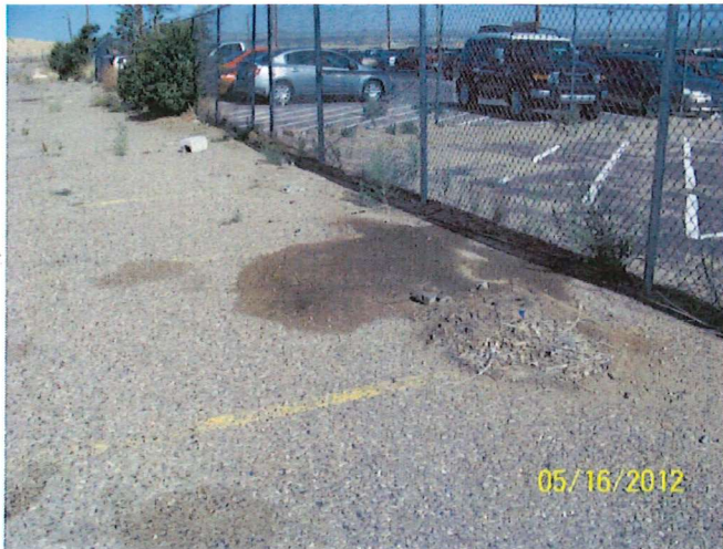
Oily staining on the asphalt inside the fenced compound.
