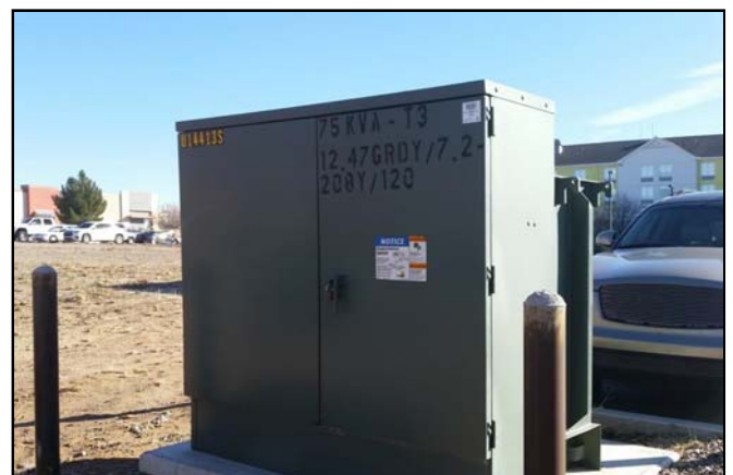
Picture 6 – View of the pad-mounted transformer located near the northwest corner of the Property.
